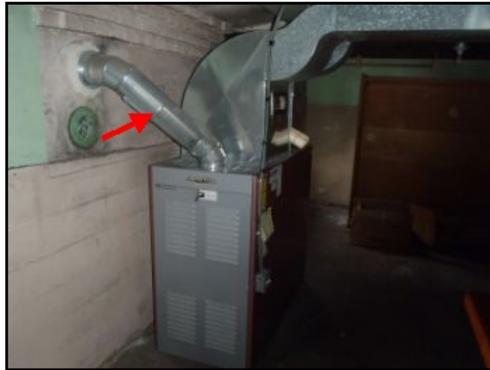
A barometric damper is missing in the exhaust vent system. Recommend repair.
