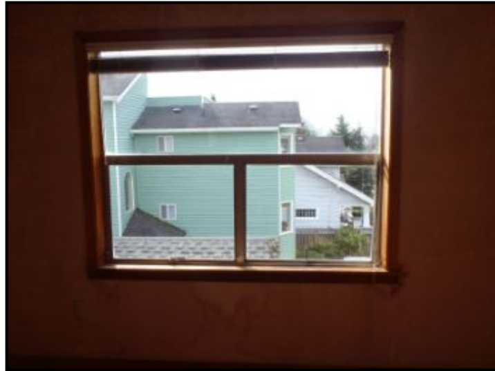
Rear upper bedroom window does not shut properly.
