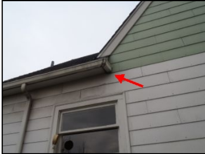
Gutter leak noted on left side of the house.
