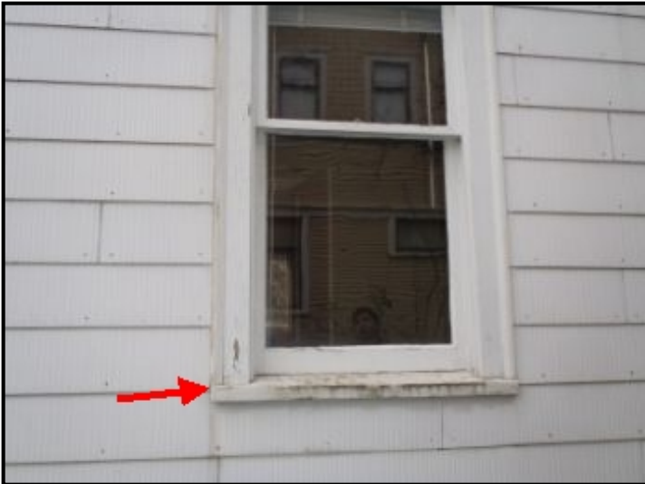
Split Caulking and peeling paint noted around all windows.
