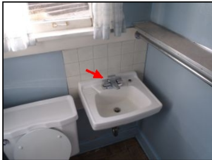
Poor pressure flow from the sink faucet.
