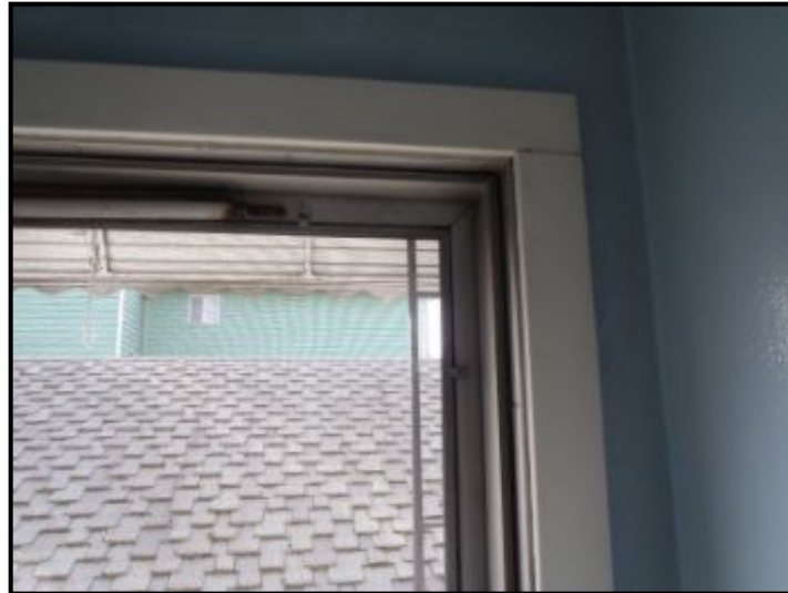
The rear patio door is missing weatherstripping.
