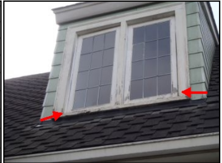
Deteriorated frame(s) at a number of upper windows.
