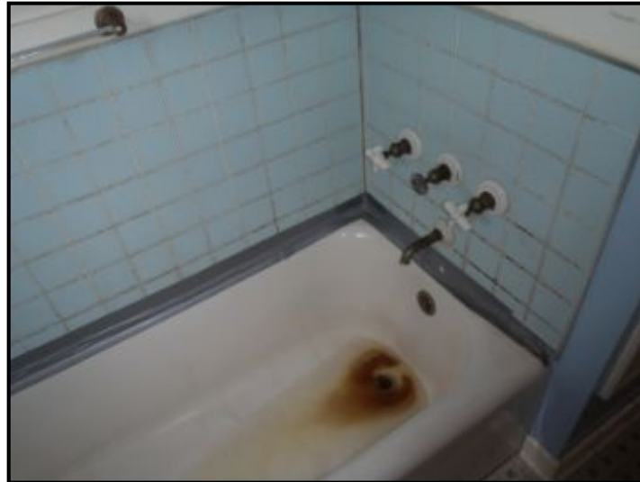
There is no water functioning in the bathtub.
